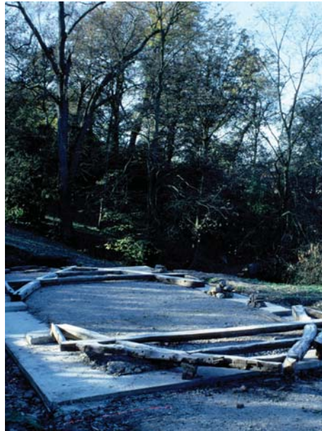
The cruck frames were drawn and numbered, then carefully dismantled and brought to Park Hill. The plan of the Barn was also recorded.
