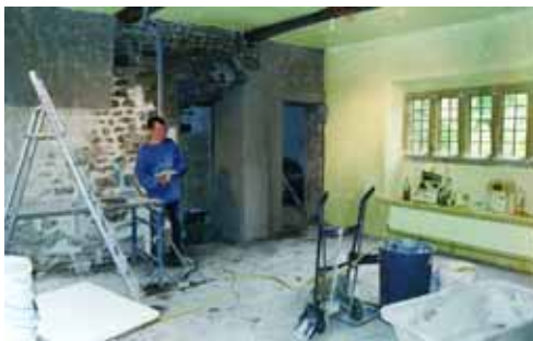
Lime plaster being applied to the wall at Pendle Heritage Centre. Three layers were required before the final yellow limewash was applied.
