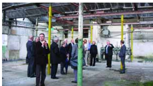
Visit by English Heritage Commissioners to Whitefield Weaving Sheds, Nelson, May 2006. The Sheds were acquired by the Trust in 2000.
